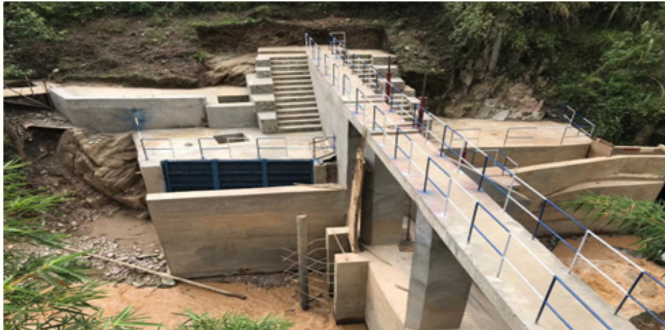
East African Pwer de Kigali – RWANDA
